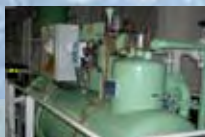
Larger bilge tank storage
